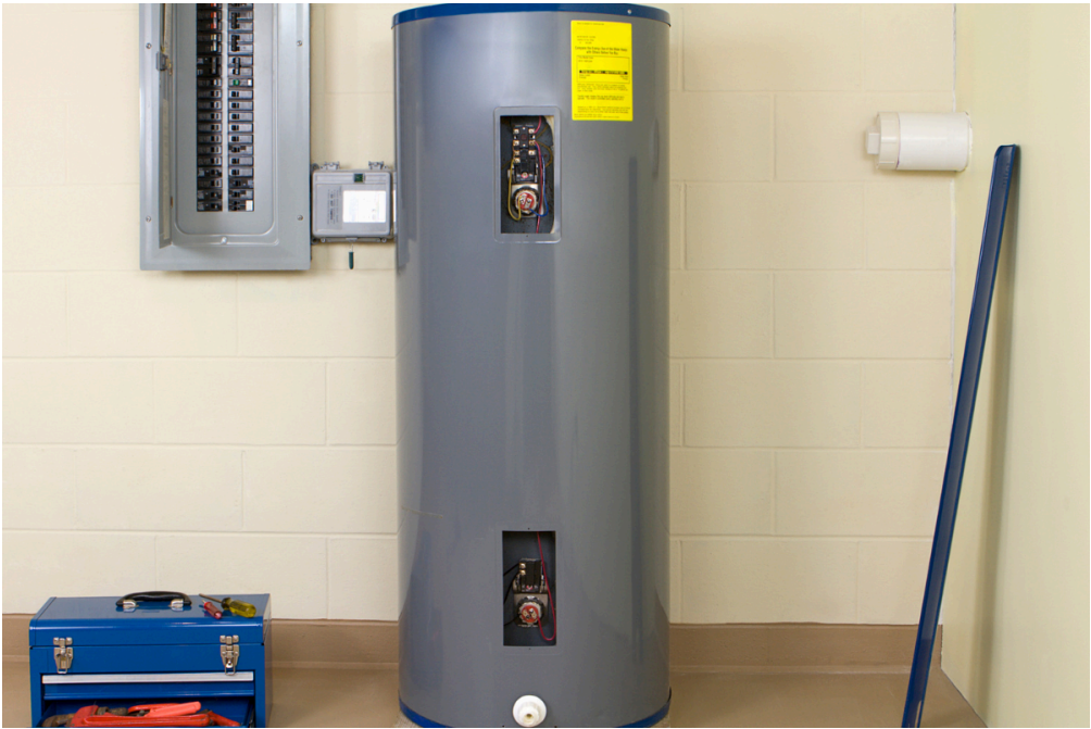
Chicago incentives preparation. Winter months assaults in ruptureds, pipes agreement, and any kind of weak point in a water heater turns up at the most awful possible moment. I have seen 5 a.m. no-heat hire January where the concern wasn't the heating system whatsoever, however a hot water heater flue obstructed by frost or a pressure relief valve frozen by a slow, unnoticed
