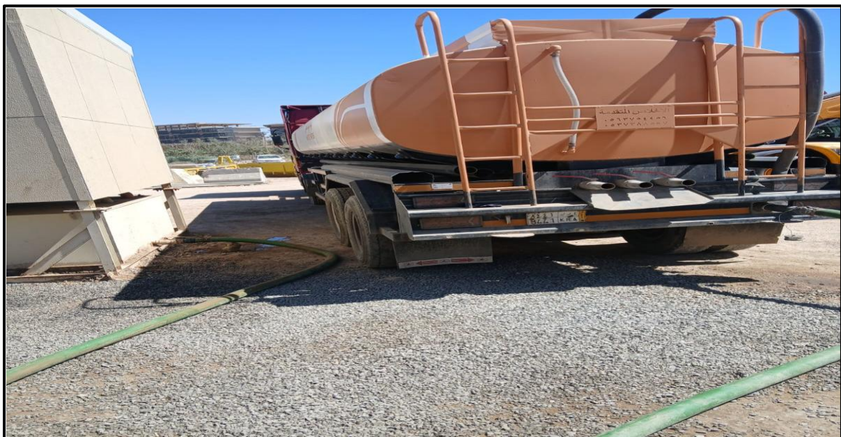
The sewage tank bund wall can be easily monitored for any leakages and damage.
